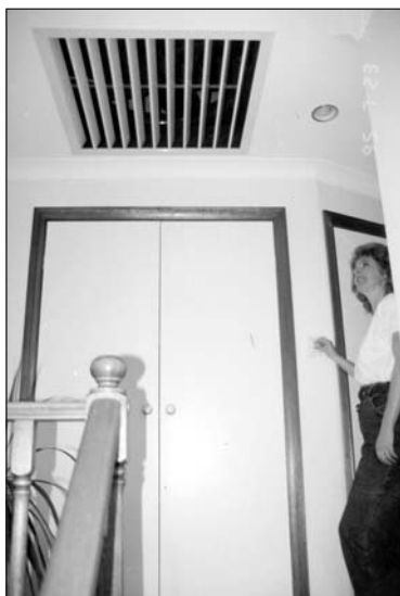
A Breeze Power Whole House Fan system installed at the top of the stair case of a two storey home.
